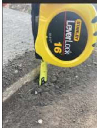
Figure 4. Trip hazard: 2 inch sidewalk crack
