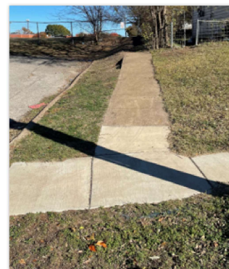
Figure 9: Sidewalk abruptly ends on Meadow Ln
