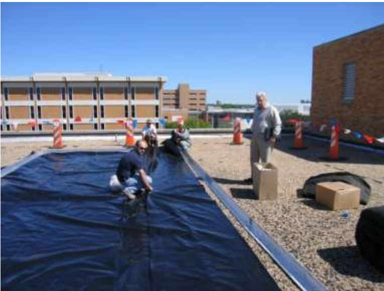
Figure 5: Installation of root barriers as Robert Nichol, of American Hydrotech, looks on
