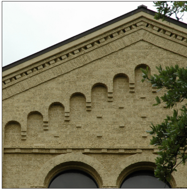
Brick articulation is encouraged as a way to create visual interest and hierarchy. Door and window lintels, sills, and floor coursing should be articulated.
