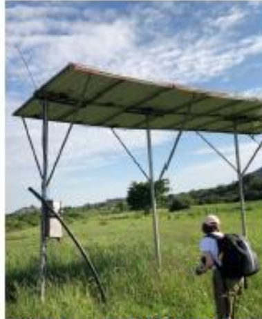
Solar panels and controller
