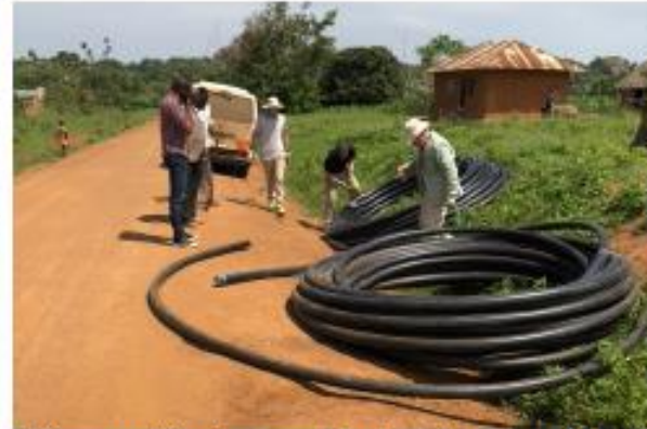
Pipes used to transport water from borehole to tanks
