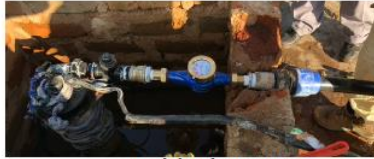
Borehole and water meter
